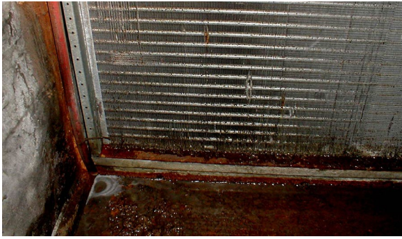
Biofilm on coil and in drain pan
